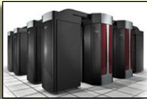
NCEP Central Operations College Park, MD (Supercomputers in Reston & Orlando)
