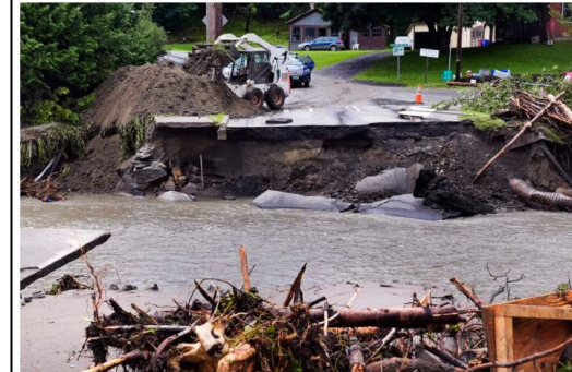
A loader dumps dirt along a washed out portion of Mill Street after remnants of Hurricane Beryl caused flooding and destruction, Friday, July 12, 2024, in Plainfield, Vt. (Charles Krups/AP)
